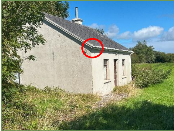
Plate 3.2 Residence (S_02) present on the eastern side of the bridge (S_01). Minor gap present between the tile and gutter.
