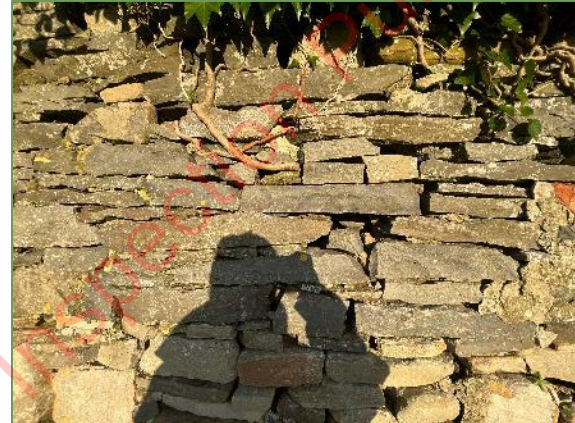
Plate 3.9d Gaps between the stonework on the gable end, providing suitable roosting habitat for individuals bats (S_09).
