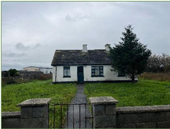
Plate 3.4 Occupied residence (S_06) with lifting slate roof tiles providing potential gaps for access.
