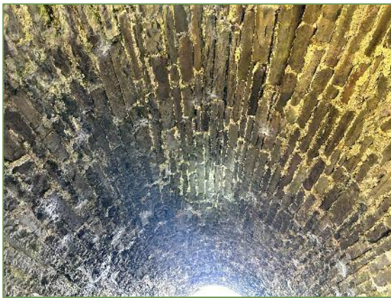
Plate 3.7e Recently pointed stonework within the barrel of the bridge.
