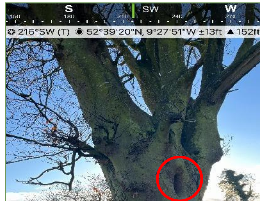
Plate 3.11 'T_05' showing signs of damage from a torn limb (too shallow to support a significant roost) and a knot-hole which may be used opportunistically by individual bats.
