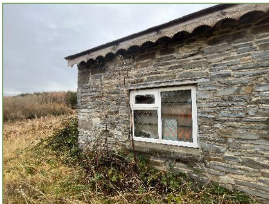
Plate 3.13b Broken window at the rear of 'S_11' providing potential access into the interior of the building.
