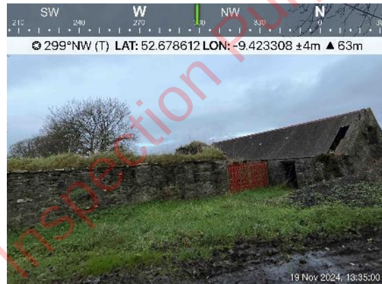
Plate 3.15 Stonework shed with asbestos roof. Large hole within the roof allowing significant light ingress (S_13).
